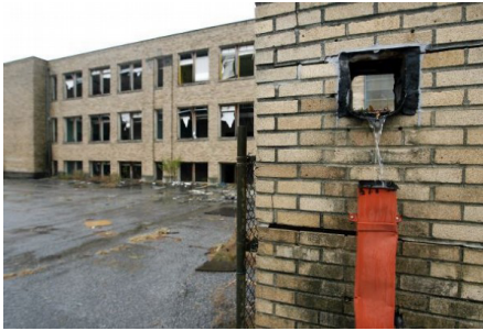
Figure 2.9 Old Manassas High School Abandoned. (Image owned by Commercial Appeal.) Photo by Dave Darnell
