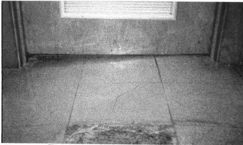
Fig. 4. Misaligned door frame due to heave in floor slab
