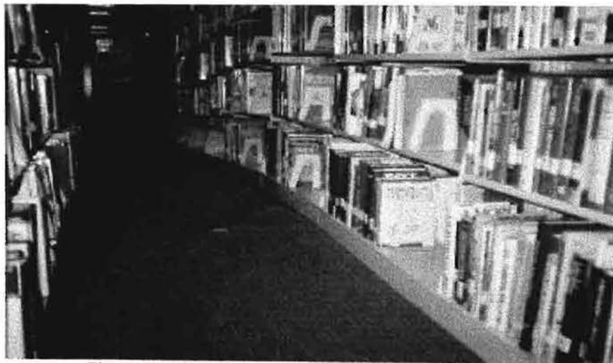
Fig. 1. Heaving of floor under bookshelves at JC library
