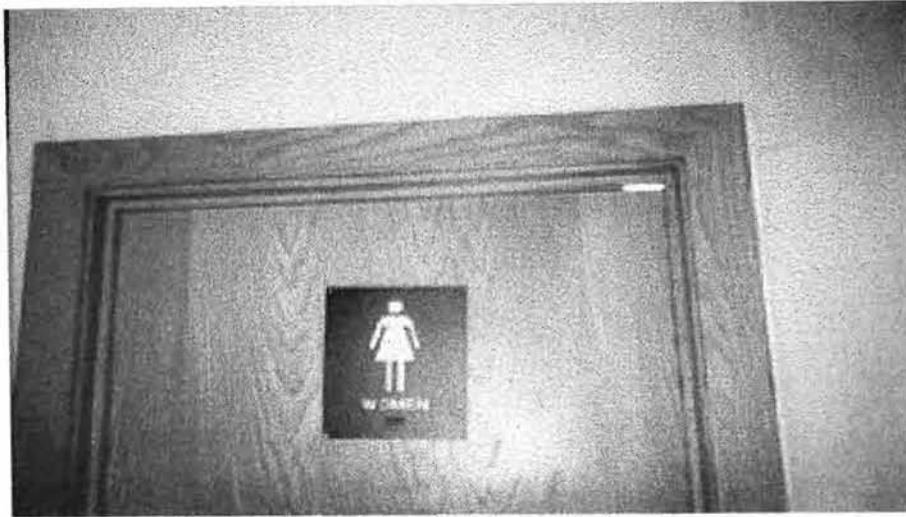
Fig. 5. Misaligned door frame at women's restroom
