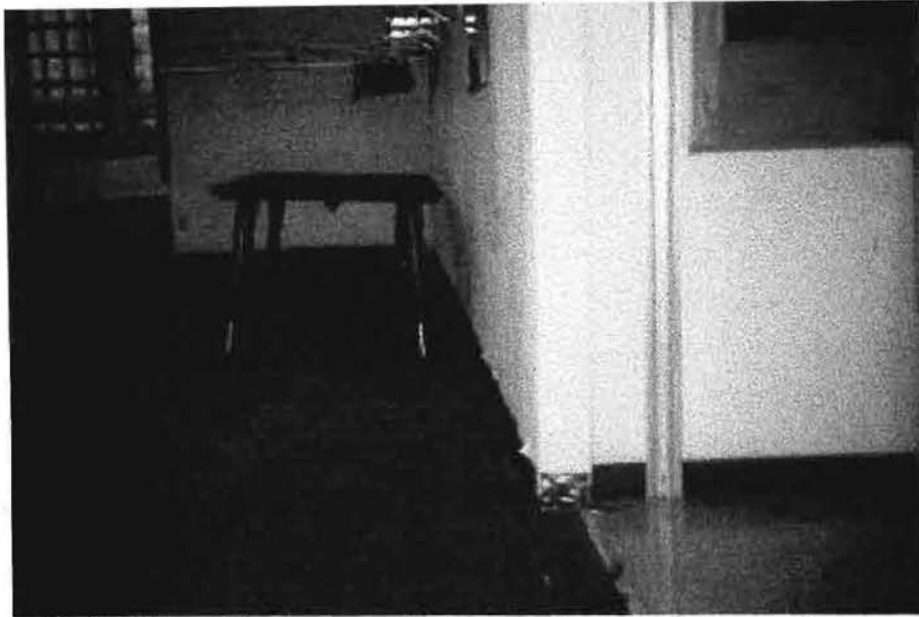
Fig. 2. Tilting of floor and separation between floor and wall in recreation room
