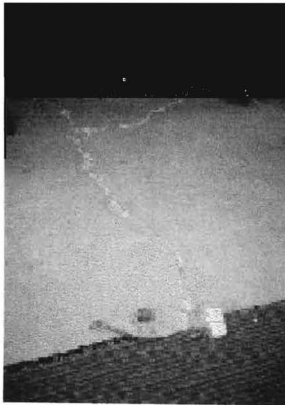
Fig. 3. Cracking of floor slab in staff area
