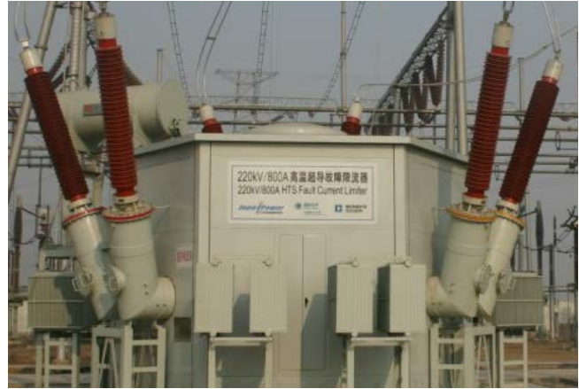
(b) 220kV SCFCL Installation
