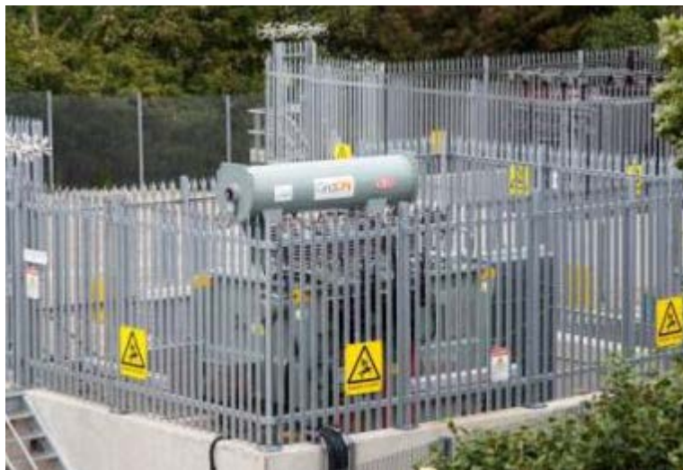
Figure 8 11kV GridOn SCFCL Demonstration [18]
