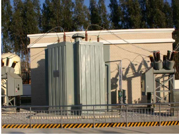
(a) 35kV SCFCL Installation
