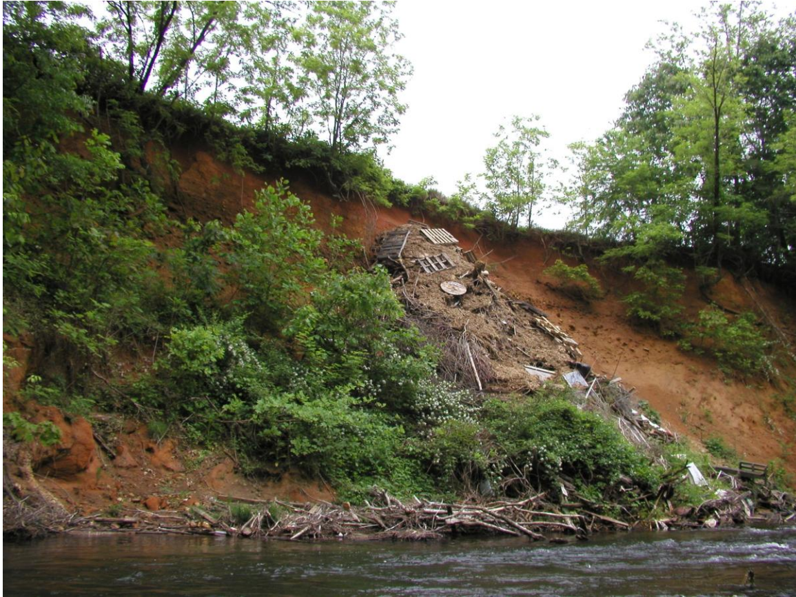
Figure 2. Eroding stream banks and an unauthorized dumpsite on the Pigeon River in Haywood County, North Carolina (September 19, 2007).
