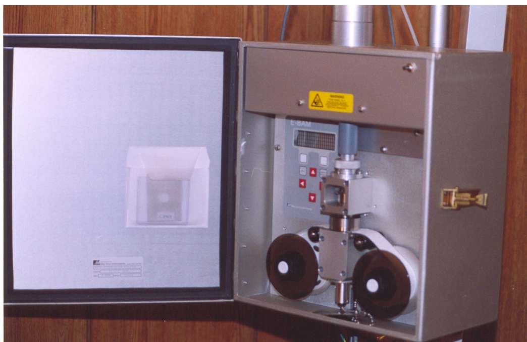
Figure 3.5 E-BAM PM 2.5 Analyzer Inside Monitoring Trailer
