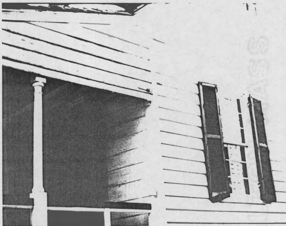
Figure 8. Noticeable damage to the historic structure.
