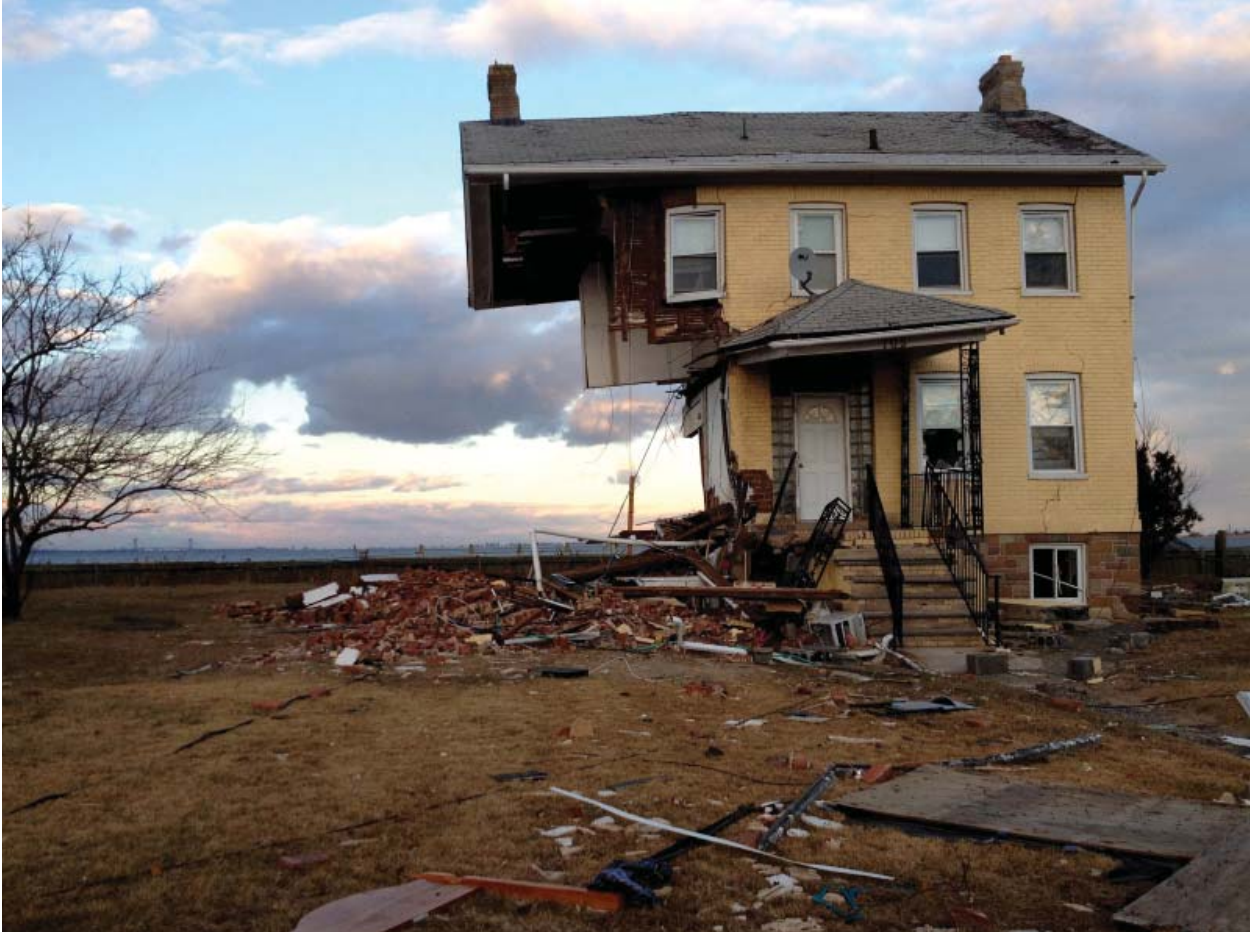
Figure 1: A House After Hurricane Sandy
