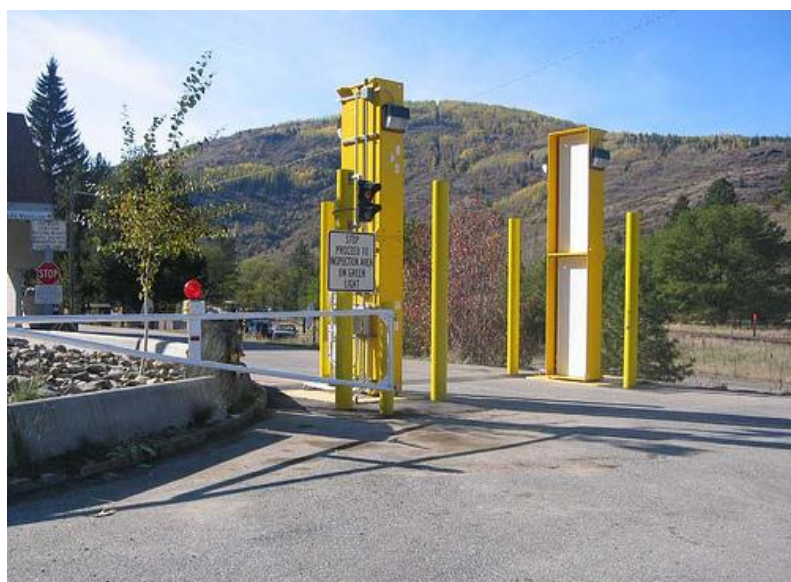
FIGURE 1 - RADIATION PORTAL MONITOR INSTALLED ALONG THE U.S. BORDER
