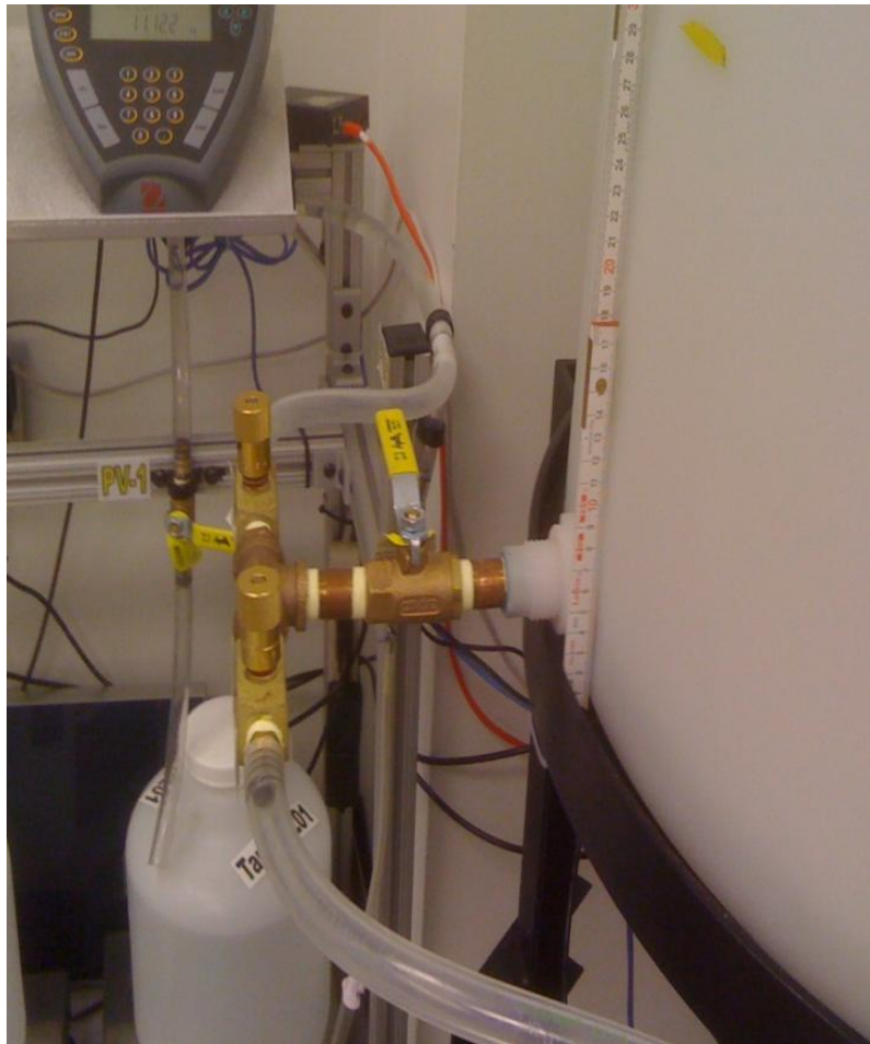
Figure 14 - Original Surge Tank Control Valve Setup
