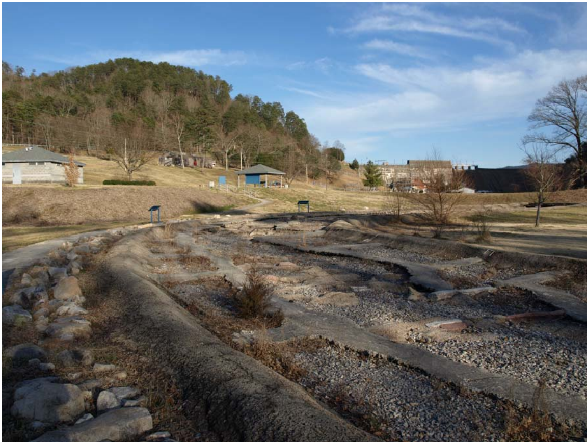
Figure 37: The Ocoee Olympic Whitewater Model is a valuable and unique feature to celebrate the Olympic games but is in needs of repair and rehabilitation. Source: Nathan Oliver
