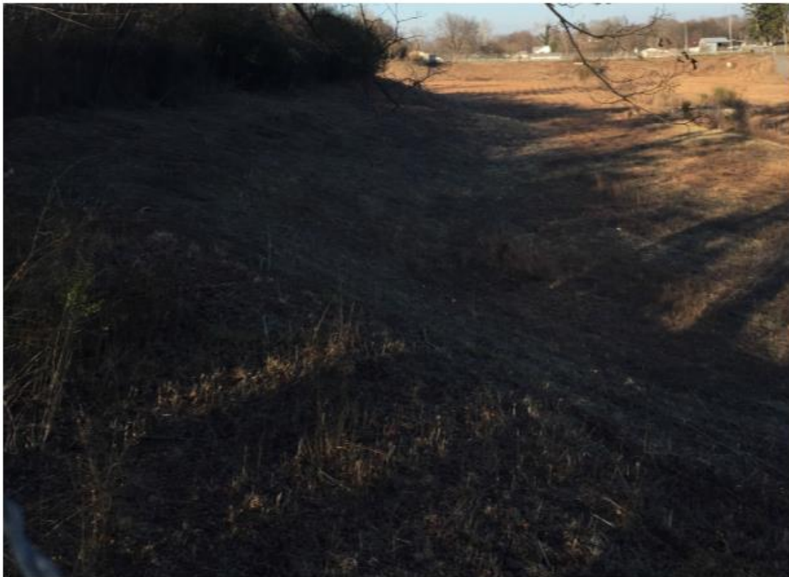
Figure 9 Steep inclines between the fence and bottom of retention pond
