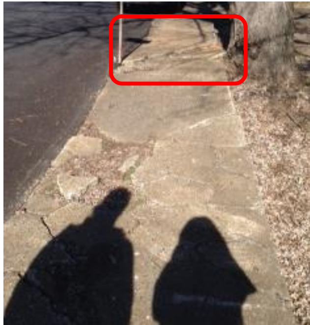
Figure 12 Cracks occurring on existing sidewalks on Blythe Avenue
