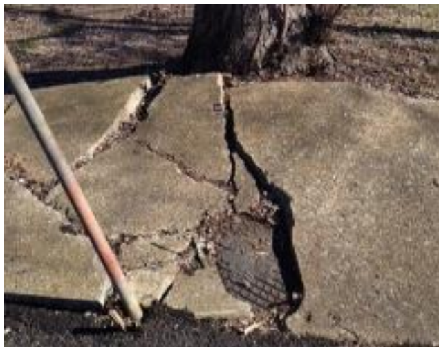
Figure 12a Close up of the cracks occurring on existing sidewalks on Blythe
