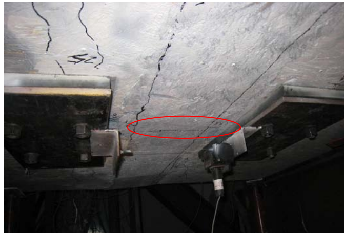
Fig. 3.18. Transverse crack in FF-7 test
