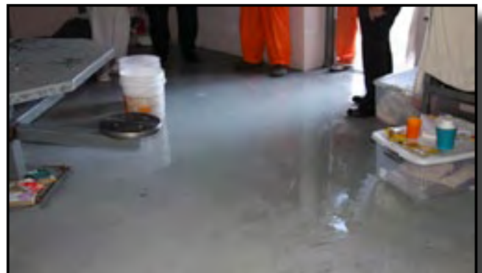
The inmates had to take shifts emptying the buckets when it rained because of major water leaks in the jail facility.
