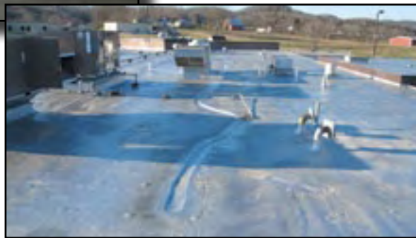
New heating and air conditioning units were installed on the new SPF jail roof.
