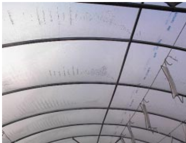
Condensation problems caused by excessive humidity levels.
